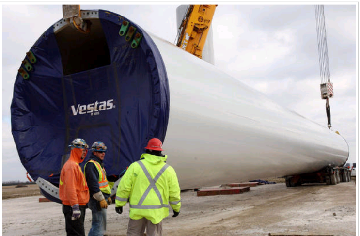
Workers accept delivery of wind turbine towers at the Pointe-Aux-Roches Wind Project in Essex County on Friday, Toronto-based International Power Canada, Inc. (IPC), a renewable energy company, is celebrating the arrival and installation of the first domestic content-compliant turbines in Ontario. (Nov. 30, 2010)
